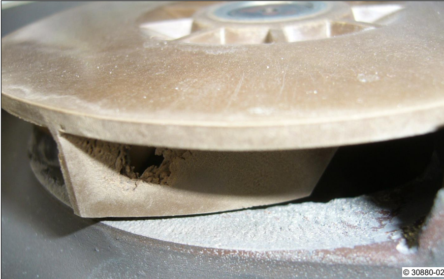
A15: Flywheel of the coolant pump, cavitated
